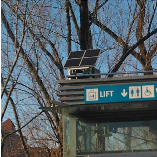
Figure 5: solar powered DIYasb box
